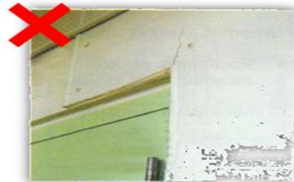
Cracks allow bacteria and moulds to accumulate
