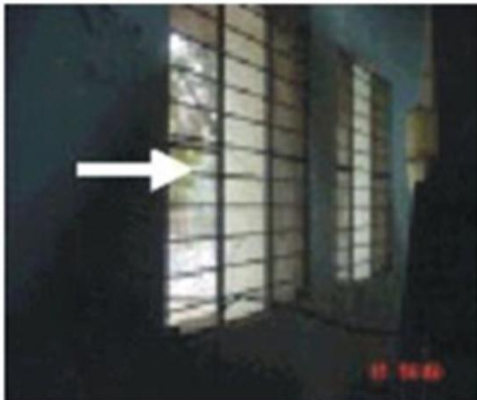
Broken glass of the window
